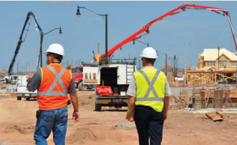
Employers and supervisors must ensure that their legal duties under the OHS and the requirements of the Construction Projects regulation (213/91) are met
