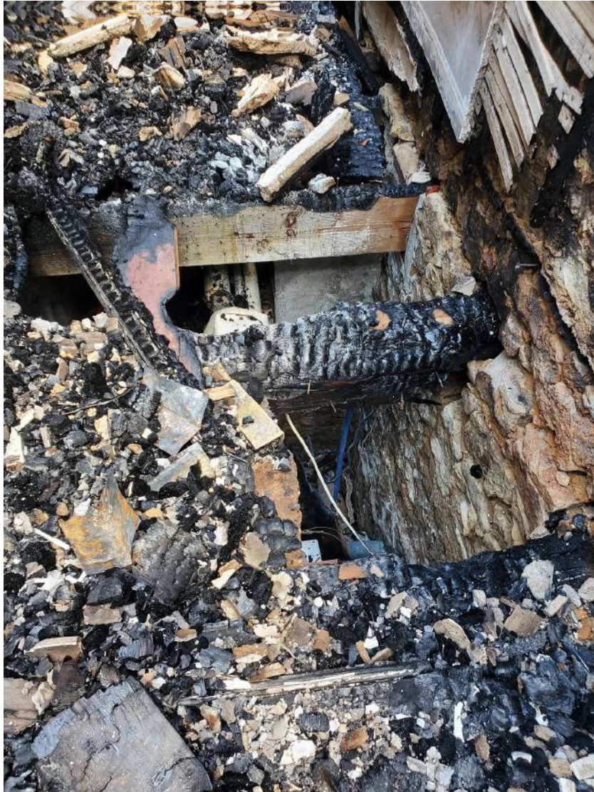
Figure 1: Typical Condition of Interior Ground Floor Framing (Over Basement) on South 2/3 of Building
