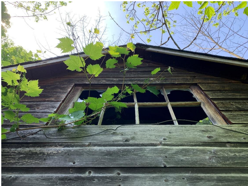
Broken window in gable end
