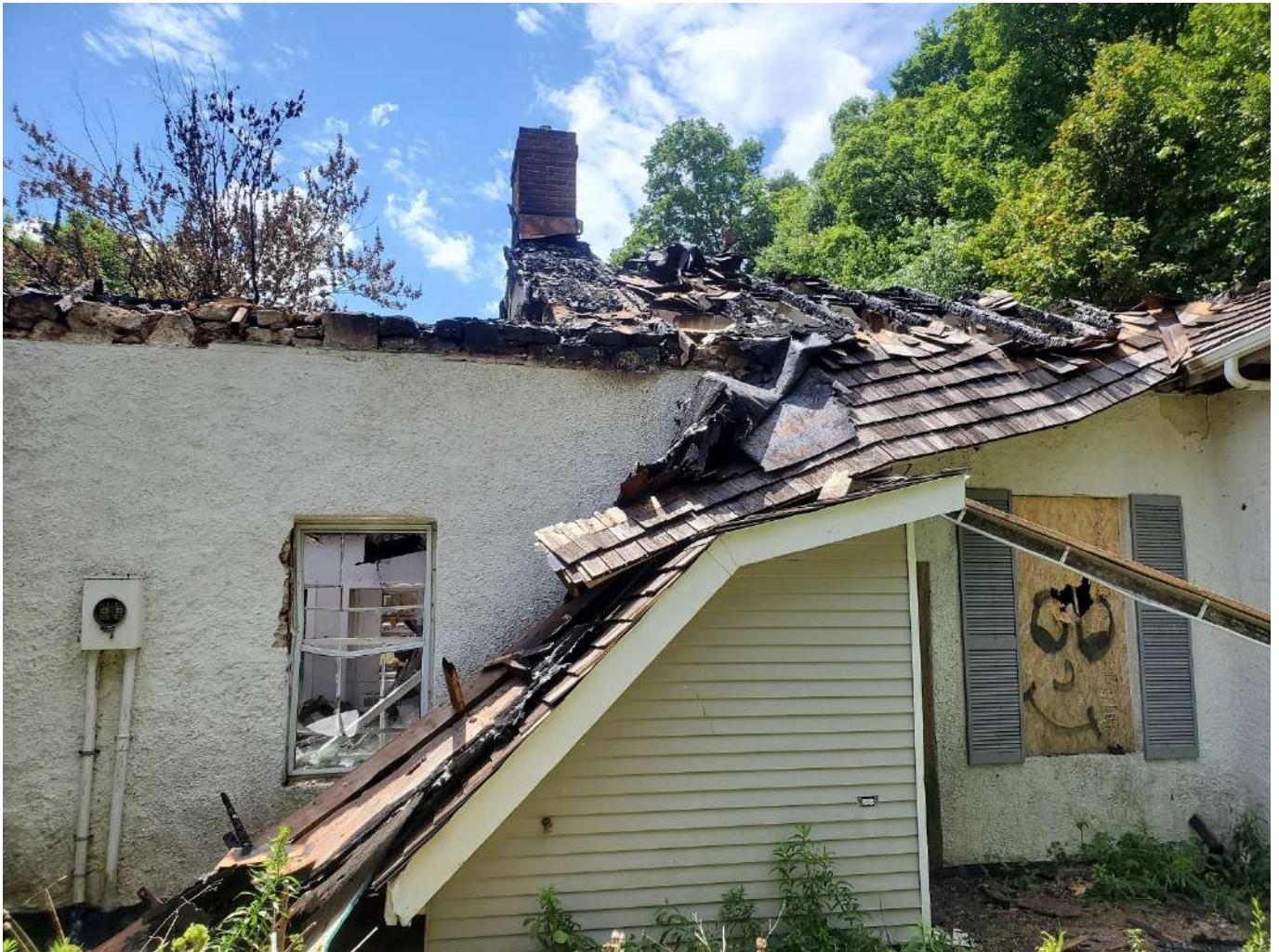
Figure 8: View From Outside of Building Looking West Showing Gutted Roof Structure to South and Fire Damage Extending Partially over North Portion of Building
