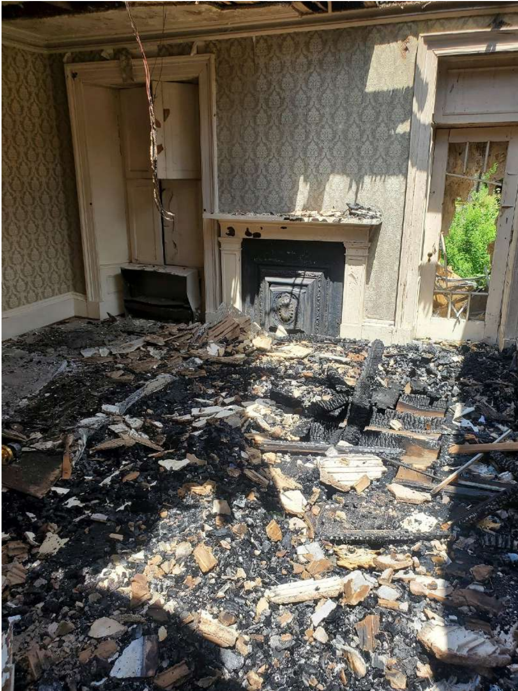
Figure 2: Typical Condition of Interior Ground Floor Framing (Over Basement) on South 2/3 of Building
