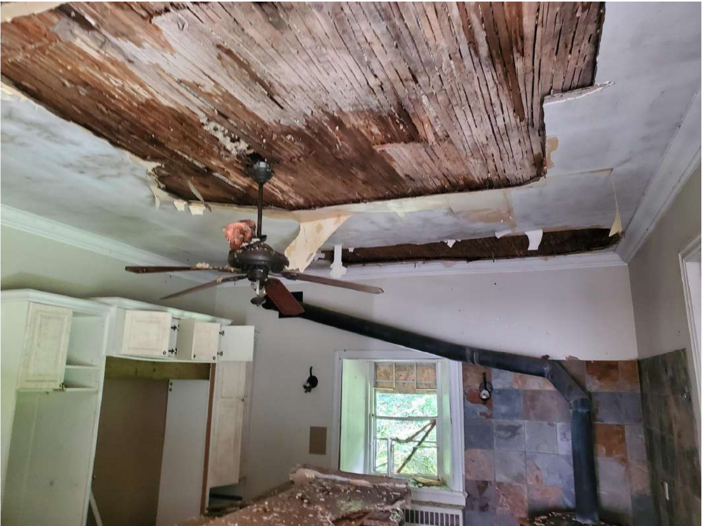
Figure 9: Water Damage to Structure in North-most Portion of Building
