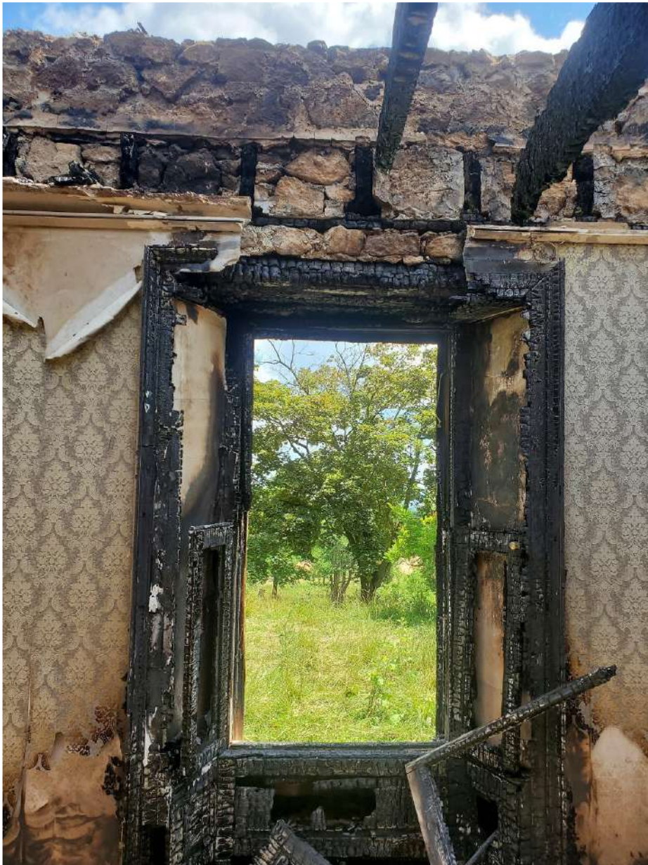
Figure 4: Typical Condition of 2 nd Floor and Roof Structure and Exterior Walls on South 2/3 of Building
