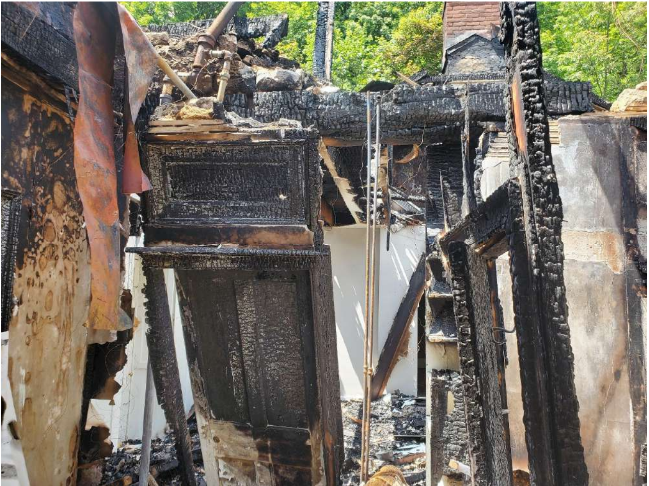
Figure 5: Condition of Much of the Remaining Interior Structure on South 2/3 of Building
