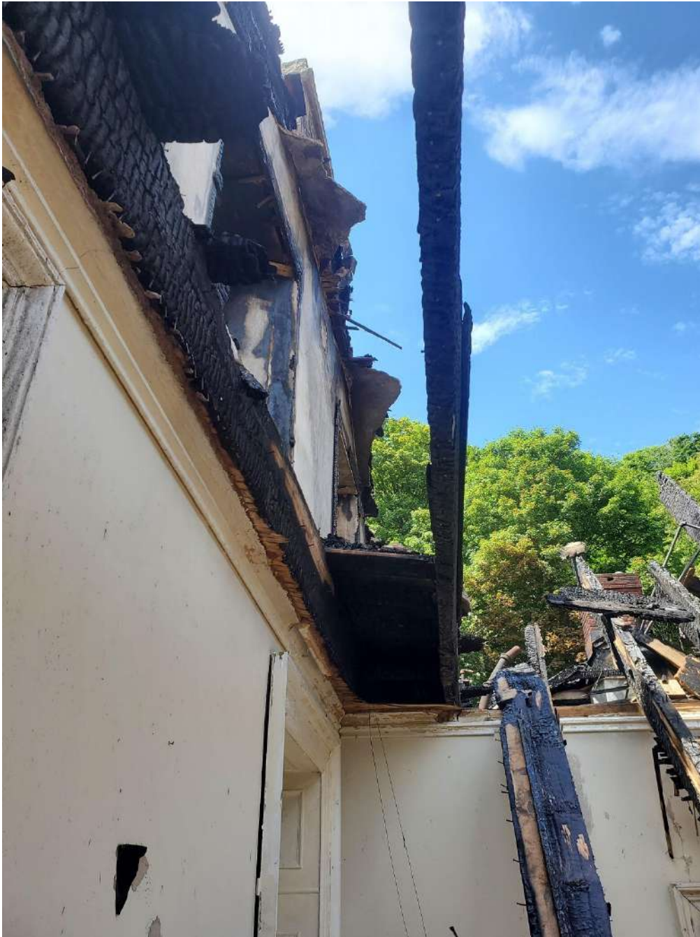
Figure 3: Typical Condition of 2 nd Floor and Roof Structure on South 2/3 of Building
