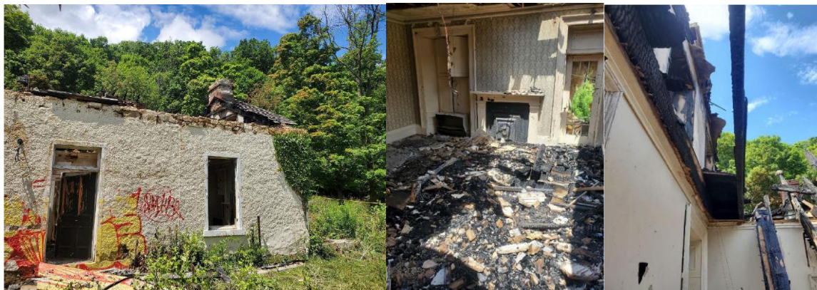
South (front) elevation shortly after the fire and interior photos.
